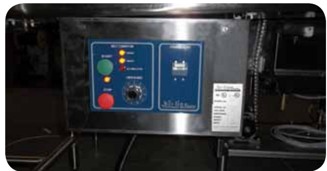
Control panel with variable speed control
