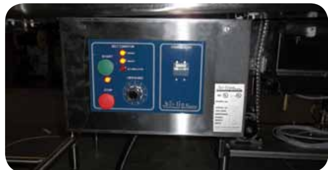
Control panel with variable speed control
